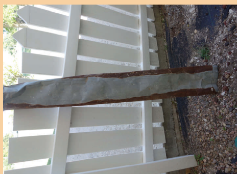
Figure 1. Old downspout extension.
