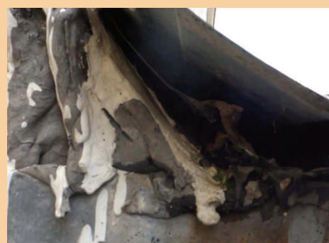
Figure 3. Gap between downspout & roof.
