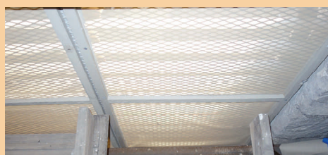
Top and Bottom Portions of a Louver with Screen Panels Attached
